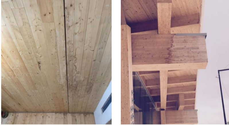
Figure 6.2 Tide marks caused by uneven leaching of extractives
