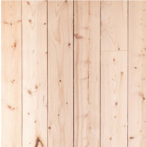
Figure 2.3 Gaps between adjacent lamination edges in a face layer
