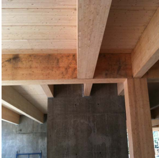
Figure 6.1 Concrete stain left when concrete is poured above
