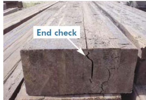
Figure 4.6 Types of checks, from APA EWS Technical Note: Evaluation of Check Sizes in Glued Laminated Timber, Form R475 .
