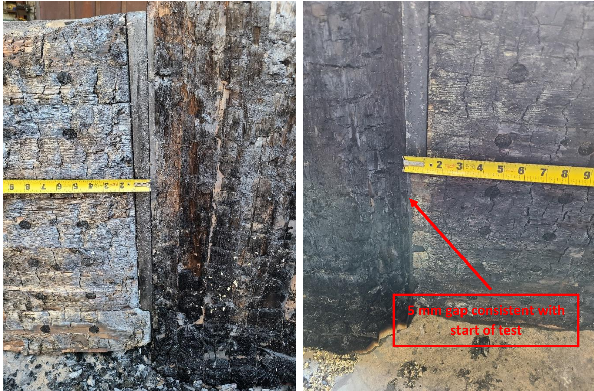
Figure 17: Photo showing remaining wood at end of beam on each side. The areas where wood remains between beam and column is consistent with the end gap of 5 mm between beam and column.
