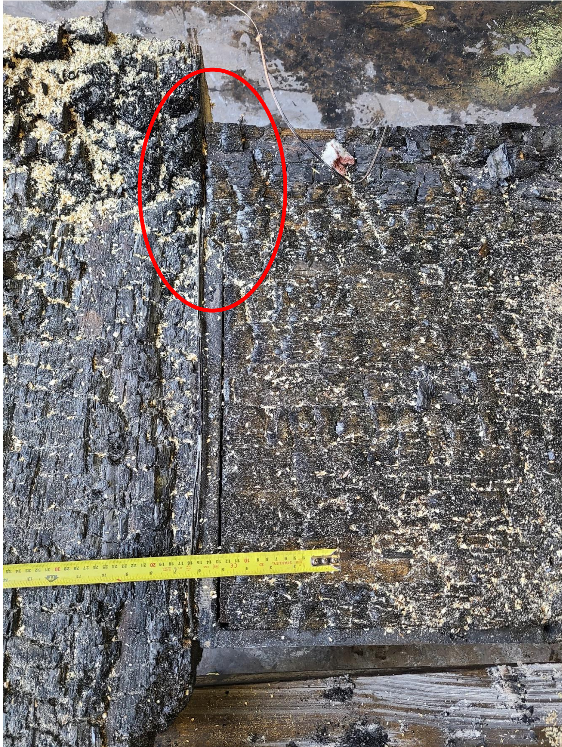
Figure 32: Remaining cross-section of beam with small amount of wood showing 3 mm gap did not expand significantly.
