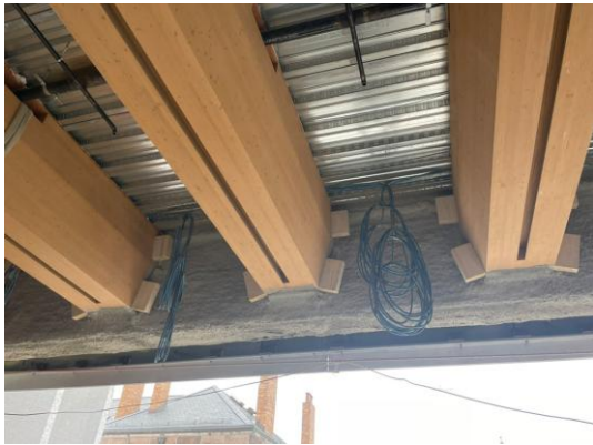
Figure 4 – Steel Structure with Cement-based Fire Protection
